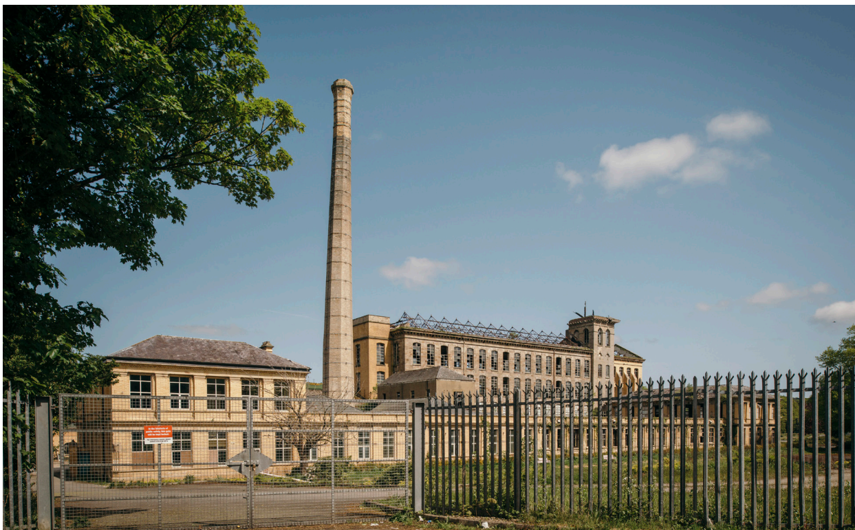
The Herdman's Mill complex ceased spinning linen in 2004. A subsequent change in ownership has failed to find viable, contemporary uses, leaving this major heritage asset vacant, physically deteriorating and vulnerable to arsonists.
