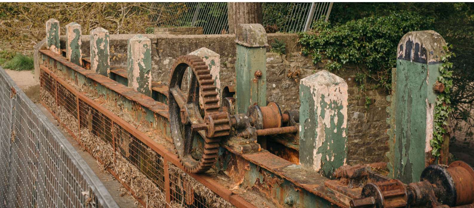
Promote the industrial heritage of the village - for instance, providing much needed maintenance to this sluice gate
