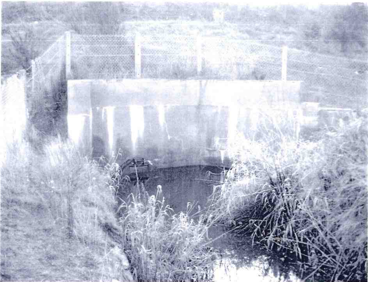
Plate 3 Flap Valve on Downstream end of Strabane Railway Drain
