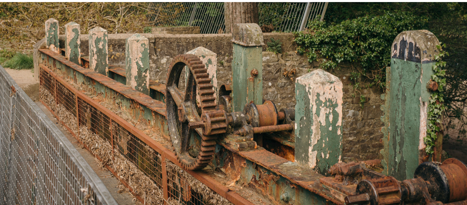
Promote the industrial heritage of the village - for instance, providing much needed maintenance to this sluice gate
