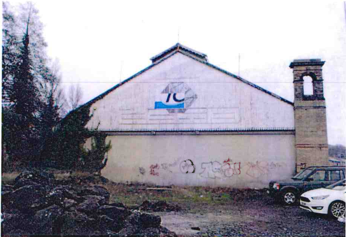
Rear Elevation to North – Timber to Upper part / Ground infilled with block
